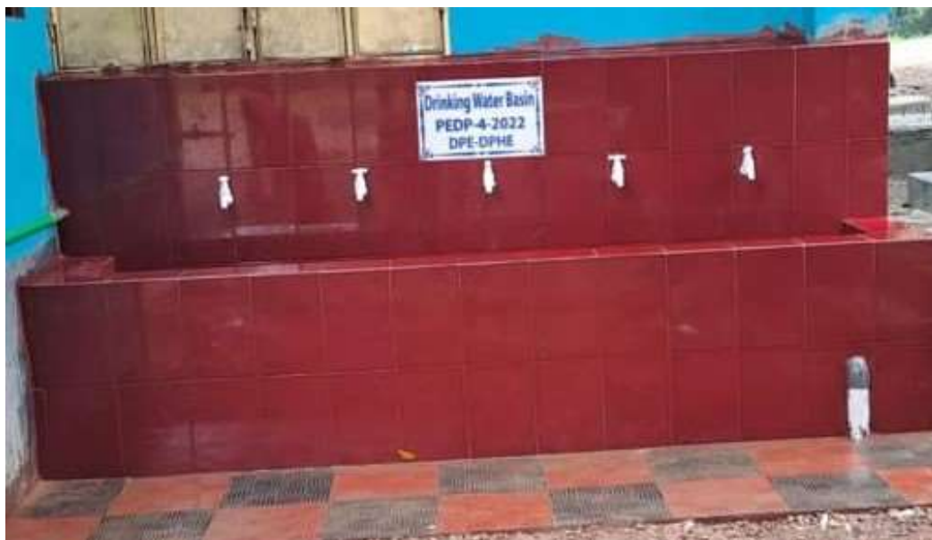
Fig. 10 Five Outlet Water Collection Basin
